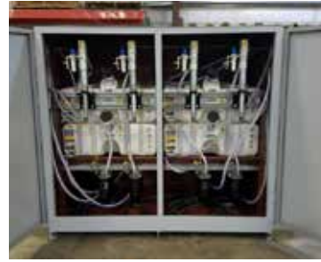
LUBRICATION FILTRATION CABINET- 4 UNIT PLASTIC - AIR
