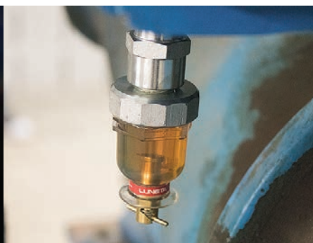
Large Blower - Wastewater Treatment Plant
